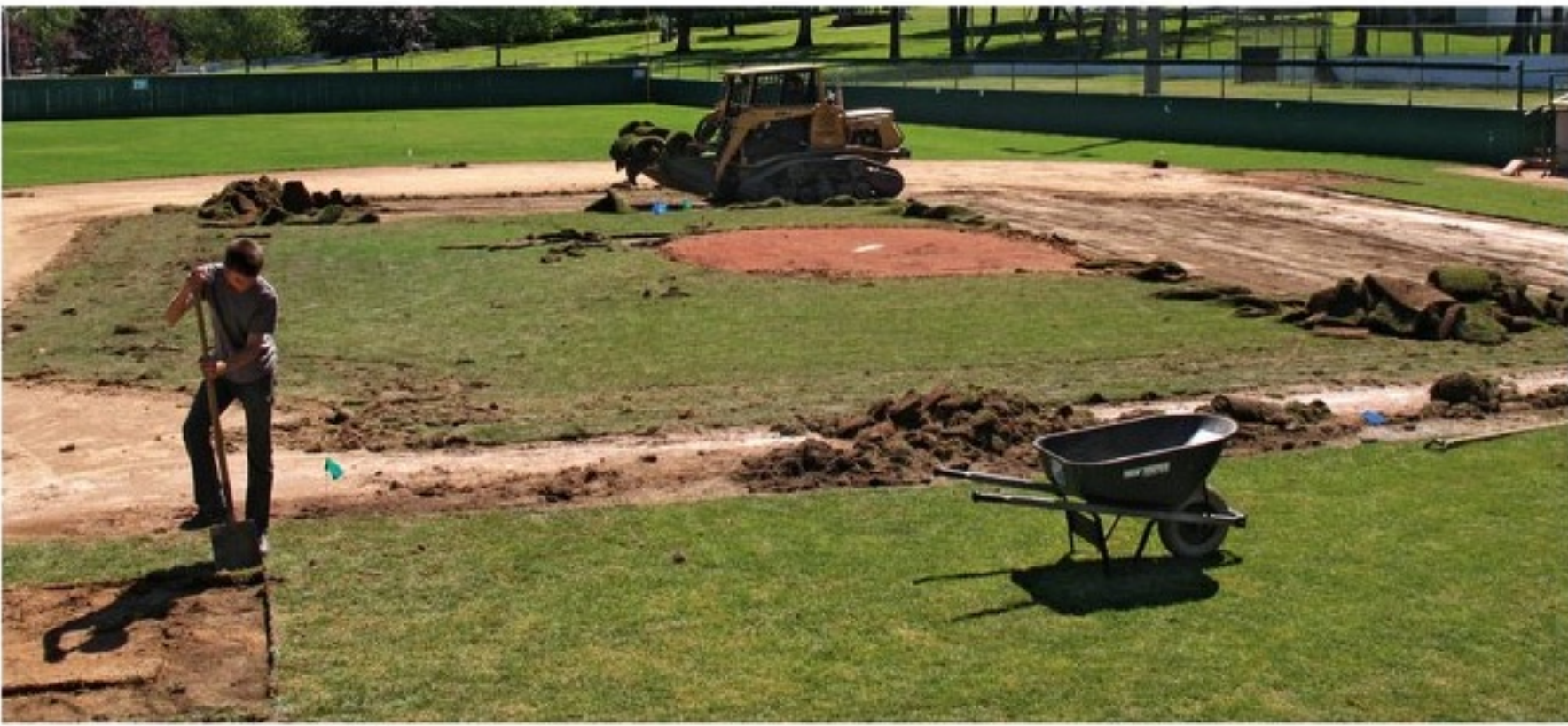
As the sod was stripped away, it was loaded onto a rubber-track loader.
