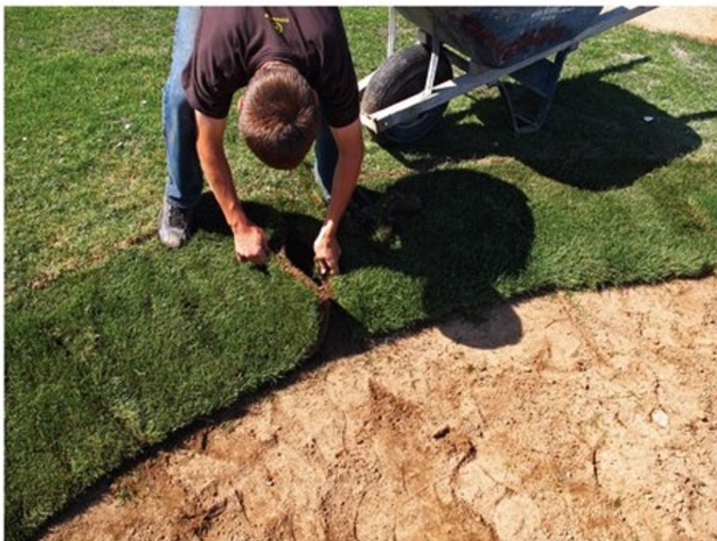
The infield turf was cut to a 1-inch depth with the sod cutter, and then stripped away in sections.
